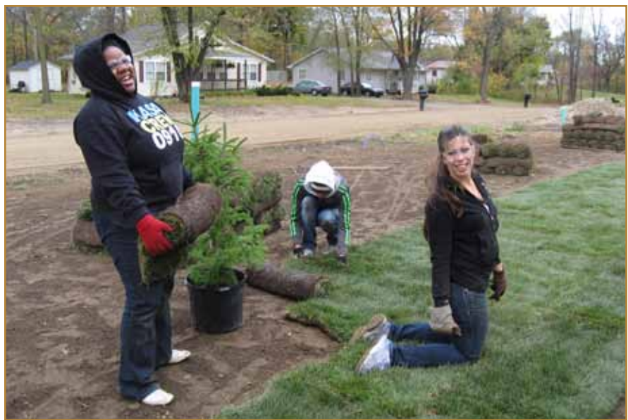
A busload of students from Andrews, comprised of Action Club members and J.N. Andrews Honors students, collaborated with Harbor Habitat for Humanity at a job site in Benton Harbor. Some worked outdoors all morning laying sod and planting trees.
